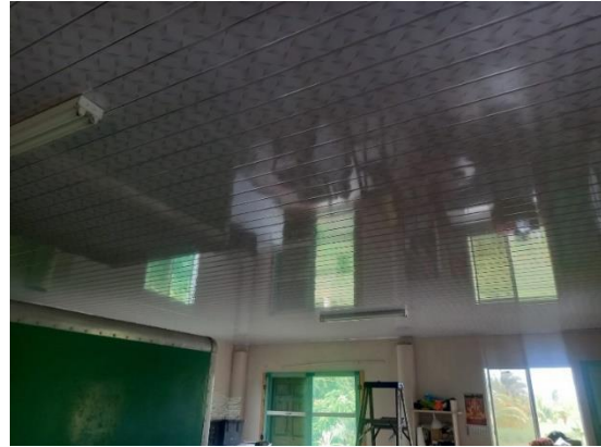
A new PVC ceiling in the agro-processing room at Nandoo’s Mango Estate ensures that all public health requirements are being met. Credit: Lonella Nandoo
