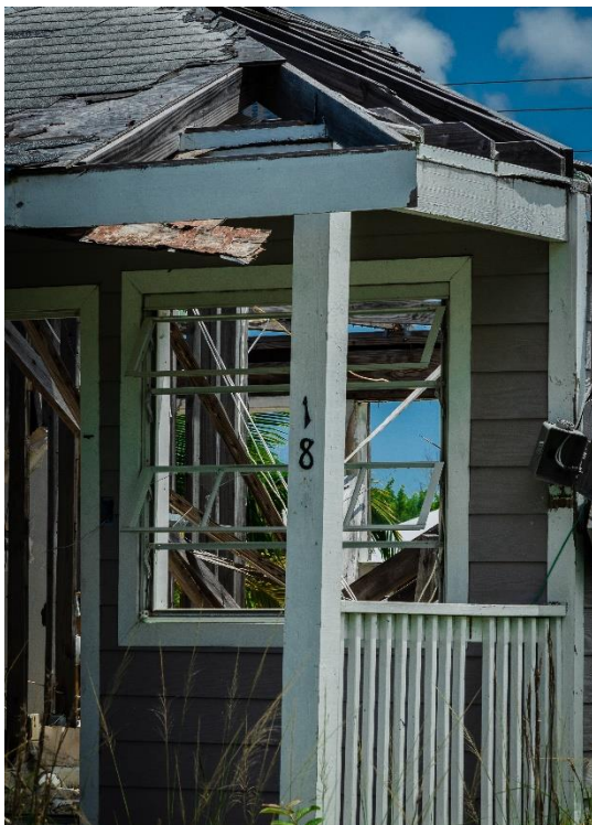
Damage in aftermath of Hurricane Dorian in Bahamas © The Heritage Partners
